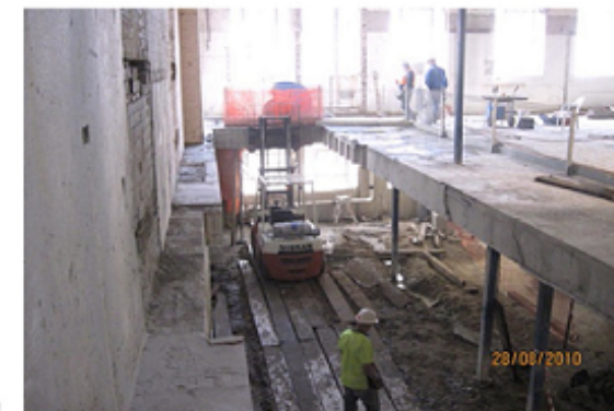
Images (top to bottom): Top - Online Concrete Cutting using the WSE1620 HF wallsaw in a floor saw application, Middle - track mounted wall saw, Bottom - Completed removal of suspended waffle pod concrete floor.
